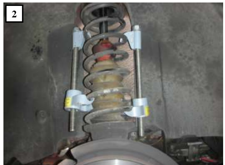
2): Using a spring compressor to “safely compress the springs. Always use a spring compressor as the compressed spring will have tremendous energy—enough to cause great injury (or worse).
